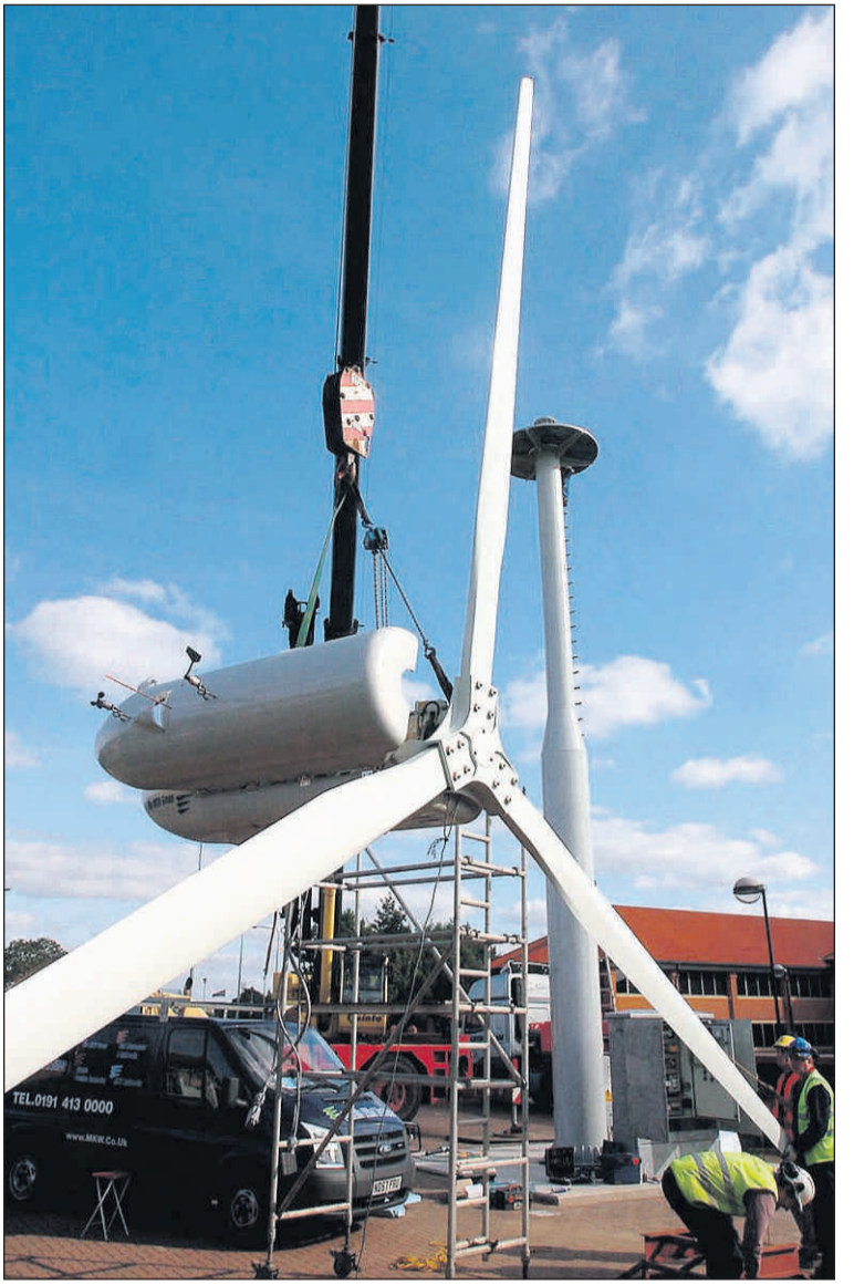
ECO EFFORT: The 13-metre-high wind turbine being erected at the new head office extension for the Mediterranean Shipping Company at Ransomes Europark in Ipswich Photograph: ANDY ABBOTT aa 08 msc turbine 1
