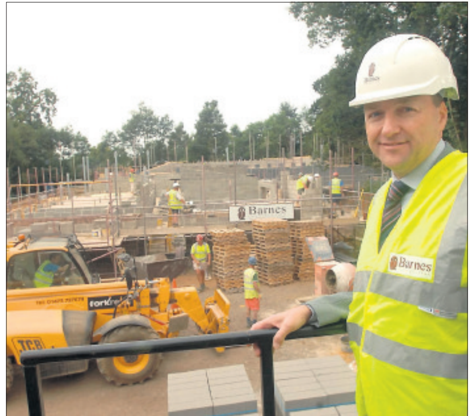
SENSITIVE: Chris Bruce, of Barnes Construction, at the hospice site where the company has erected a secure fence to prevent construction spilling over into the retained woodland
